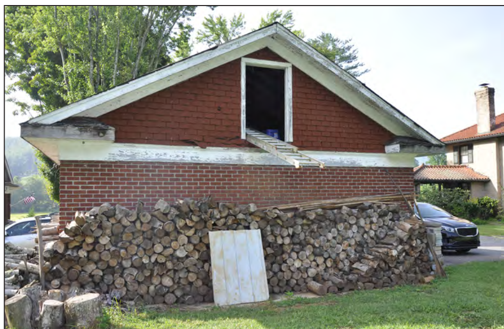
Photograph 8: View of rear (north) elevation of garage at Jeter Snyder House I; looking south. (2018)
